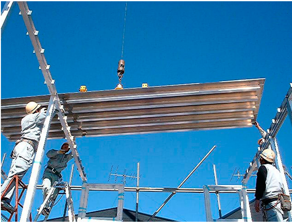
Figure 4. Aluminium components were lightweight and easy to handle on site (© Toyo Ito & Associates).
