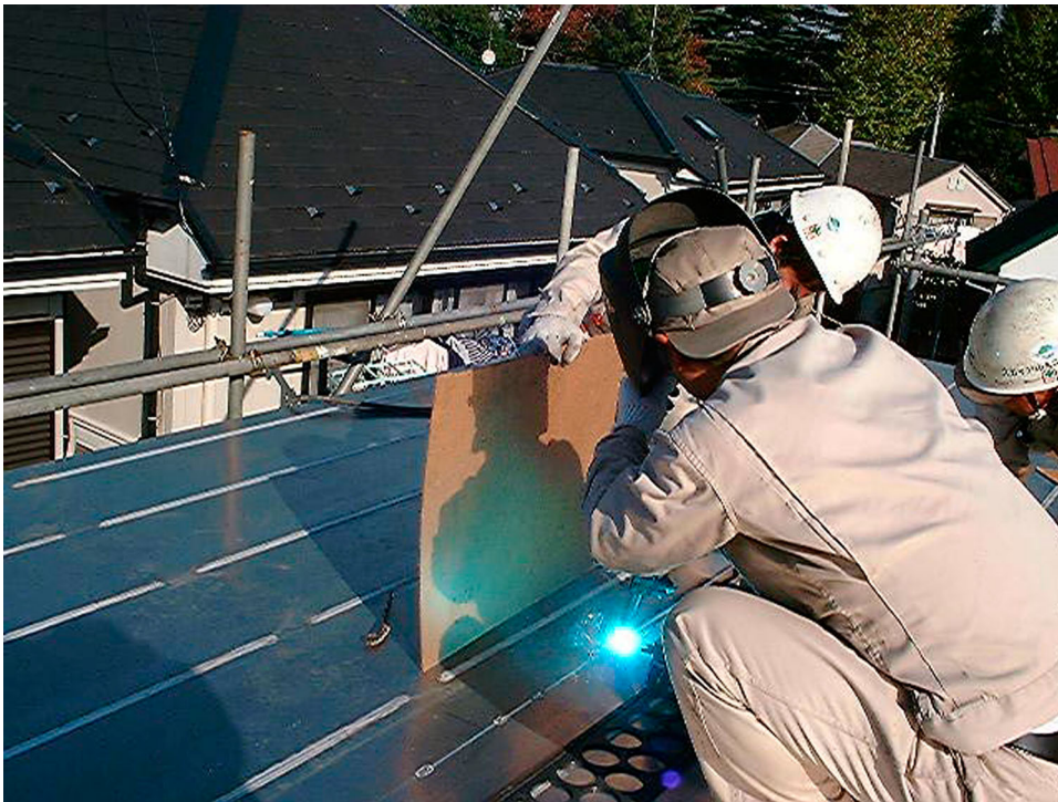
Figure 6. On-site welds were intended to create a water-resistant surface (© Toyo Ito & Associates).
